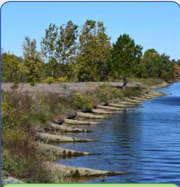
Figure 13: Living shorelines like this one along the Marshyhope Creek in Federalsburg, Maryland, protect against erosion and filter nutrients before they can enter waterways, while maintaining natural elements that benefit birds and wildlife.
